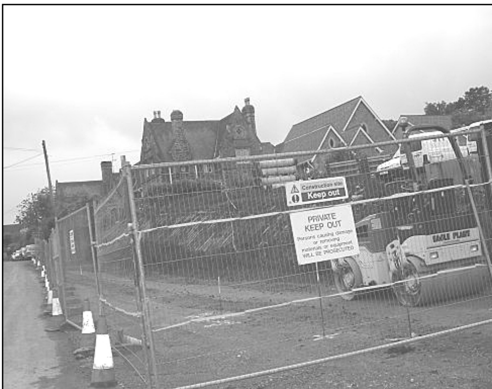
Construction of the Supported Housing - 16 bungalows for local elderly and people with a disability - is clearly under way. See Page 2
